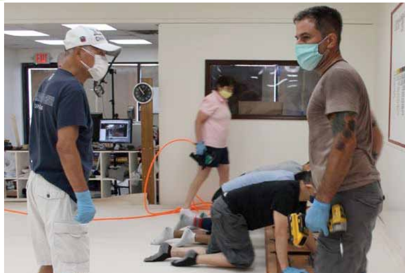
Hard at work setting up and laying the floor in the new Japan Karate & Judo Centre
